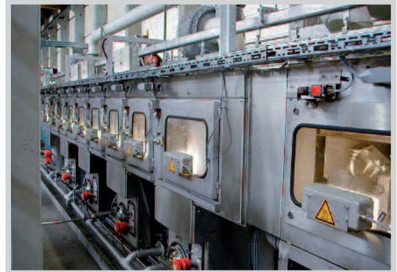
Close-up of pass-through spray facility
